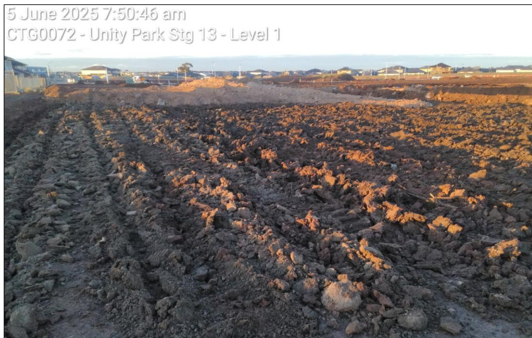
Figure 2: Subgrade Ripped (Source: C&T)
